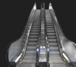
Escalators and moving walkways
