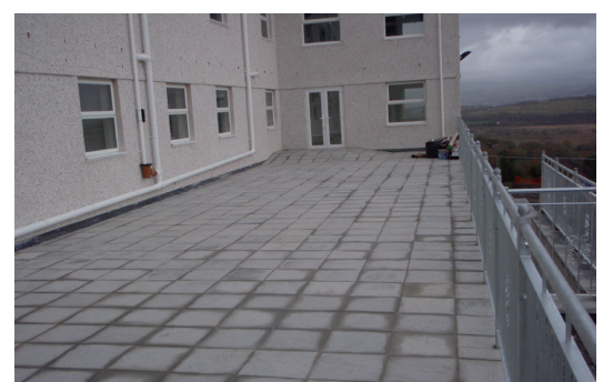
The deck finished, ready for use and fully waterproofed to protect the internal areas below
