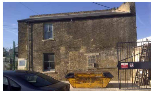
1840's Victorian end of terrace with Newtonite Lath stripped off in preparation for Diathonite application
