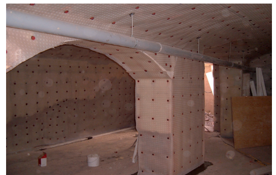
Newton 508 Mesh cavity drain membrane was fitted to the contours of the basement area, so met with listed buildings regulations
