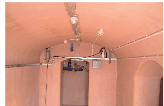
Plaster was applied directly to the Newton 508 Mesh. Newton System 500 was quick to install and trouble free
