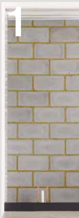
01 Once the site has been prepared, fix the aluminium site frame to the wall, ceiling and floor.
