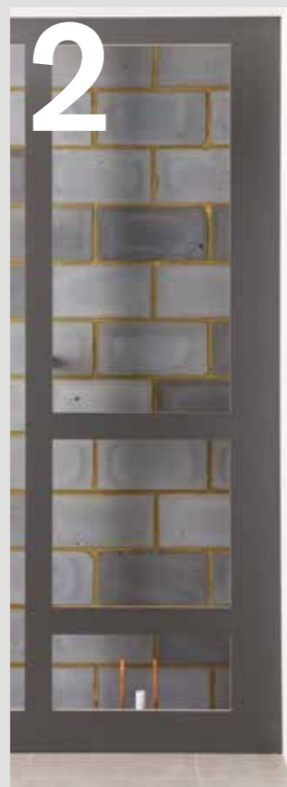
02 Fit base flashgaps to the site frame followed by vertical, horizontal and top flashgaps.
