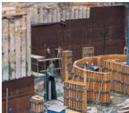
Underground garage of a Frankfurt hotel: Water emerging from the rocky subsoil is drained away by a DELTA®-MS seepage layer.
