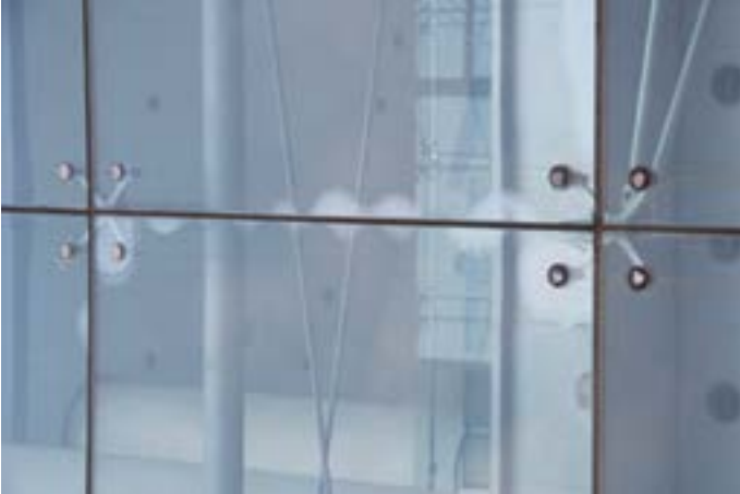
• Typical defects caused by delamination
