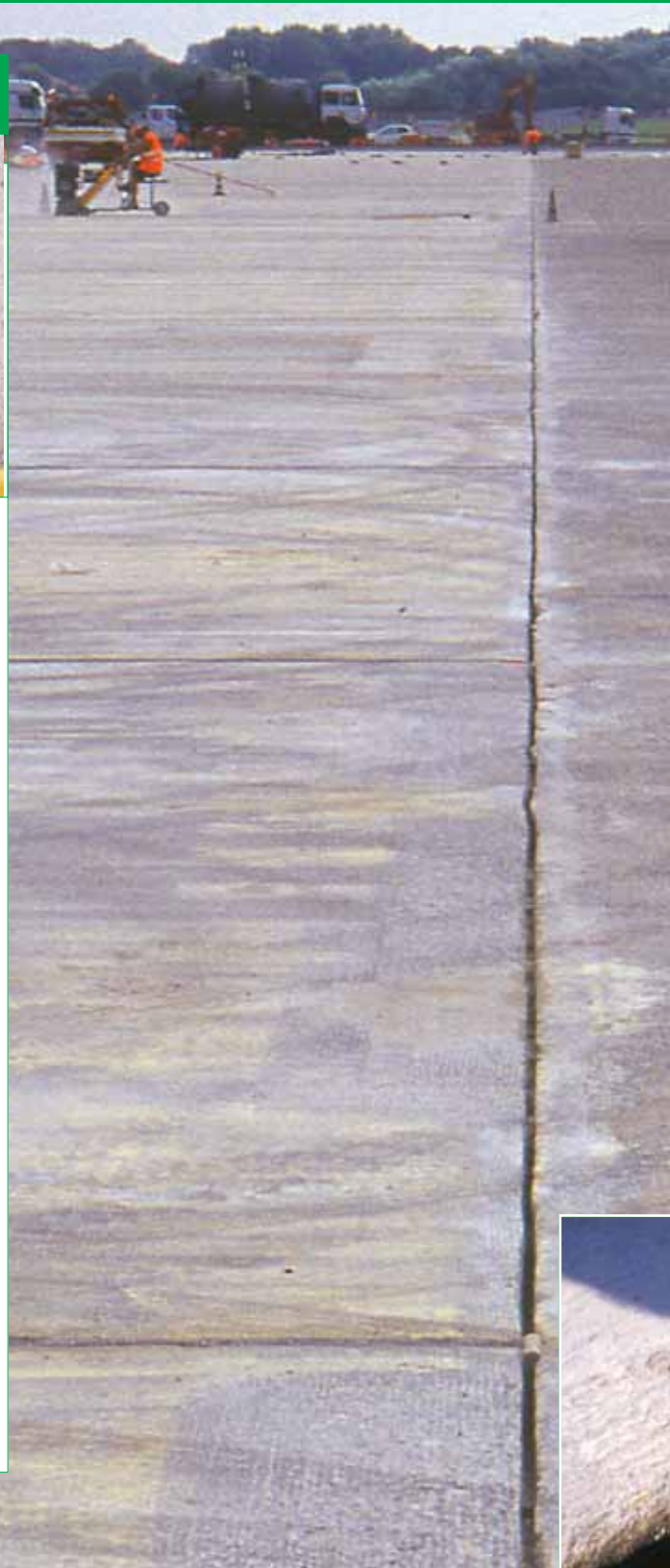
Linate airport - Milan - Italy Sealing of the runway joints with: MAPEFLEX PB27
