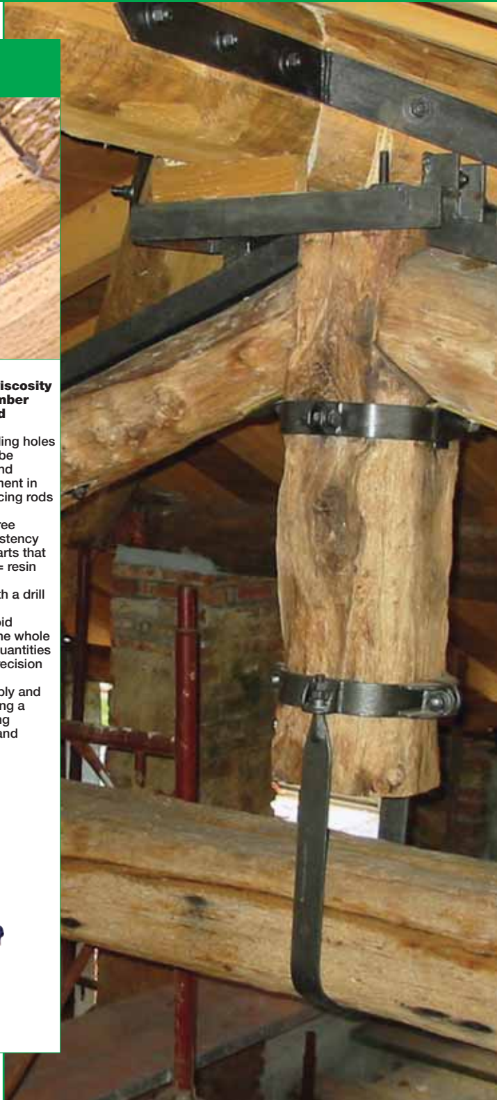
The Farmer Museum - Milan - Italy Reparation of the wooden structures with: MAPEWOOD PRIMER 100, MAPEWOOD GEL 120, MAPEWOOD PASTE 140
