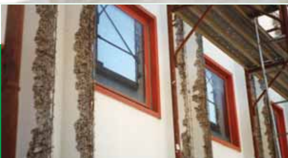
A&C Adivar Comifar industrial loft - San Nicolò a Tordino - Italy Repairation and protection of the industrial structure with: MAPEFER, STABILCEM SCC, MONOFINISH, MALECH, ELASTOCOLOR RASANTE, SILANCOLOR PRIMER, SILANCOLOR PAINT
