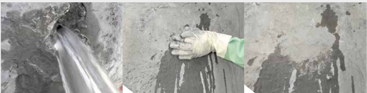
An active leakage is sealed instantly after applying KÖSTER KD 2 Blitz Powder.
