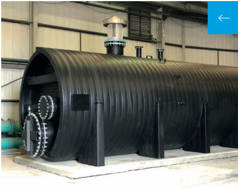
3000mm dia Potable Water Balance Tank, Broadfields, Isle of Wight
