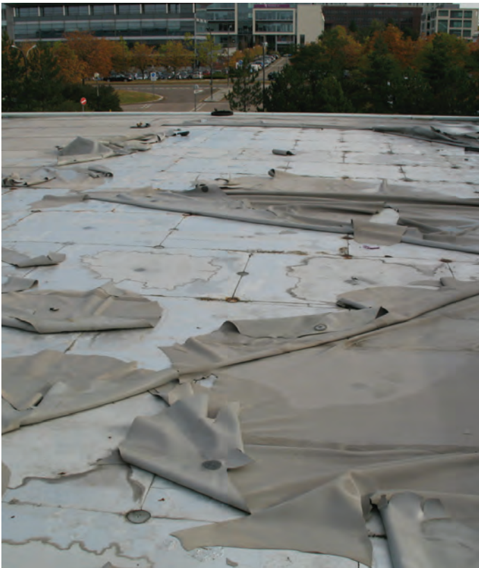
Failure due to incorrect fastener specification
