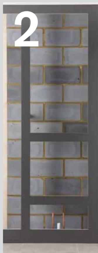
02 Fit base flashgaps to the site frame followed by vertical, horizontal and top flashgaps.
