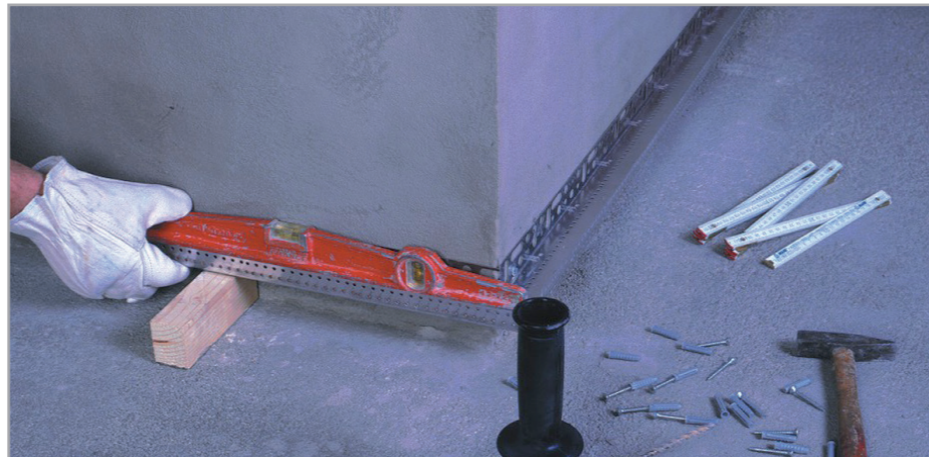
Position the support profiles: make sure they are horizontal using a spirit level
