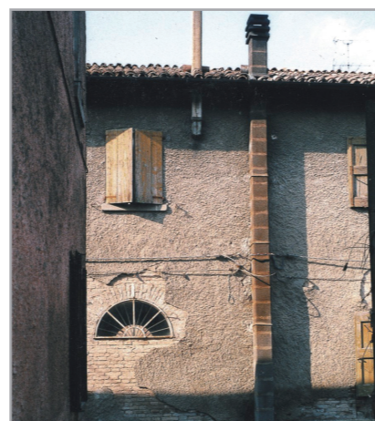
Wall with rising damp
