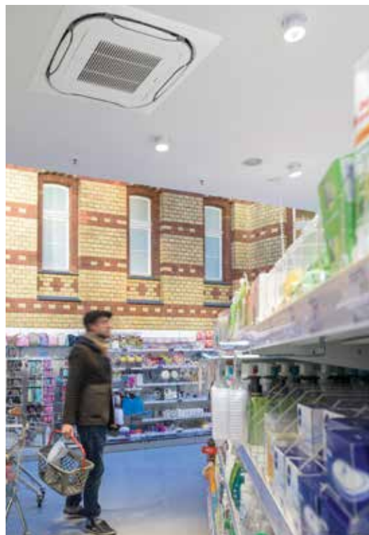
The sales area of the dm outlet is air-conditioned with six Daikin roundflow cassettes.
